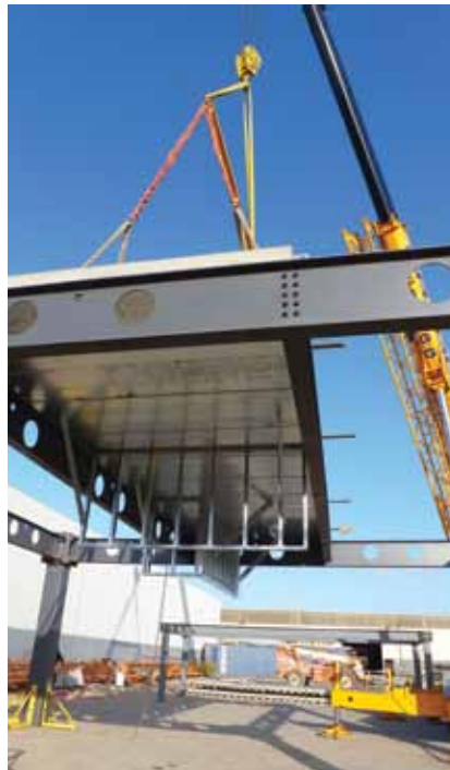
Aditazz developed floor decks as components for use in its modular strategy.
